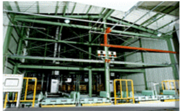
Storage & Retrieval System
